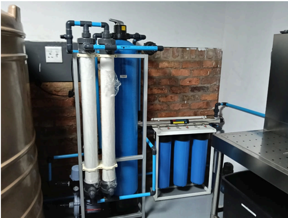
Figure A5.4: Kusini water filtration system with reverse osmosis and ultrafiltration technologies.
