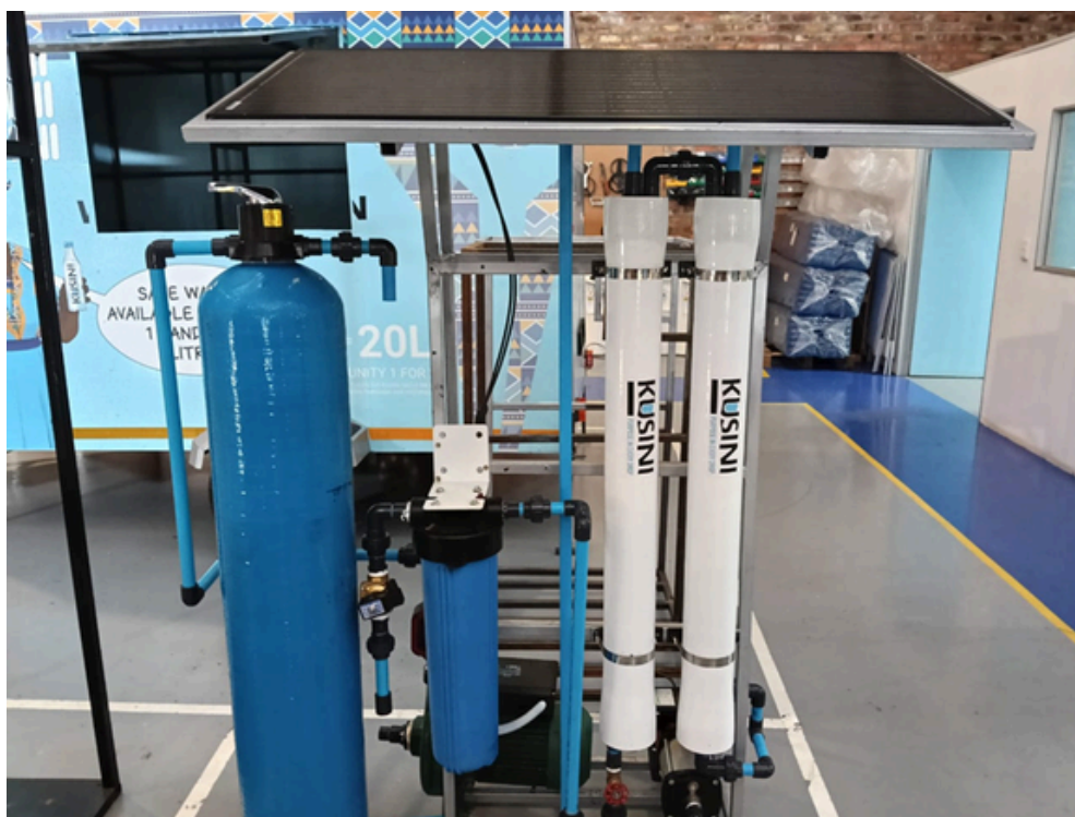
Figure 3: Kusini water filtration system combining solar, reverse osmosis and ultrafiltration technologies.
